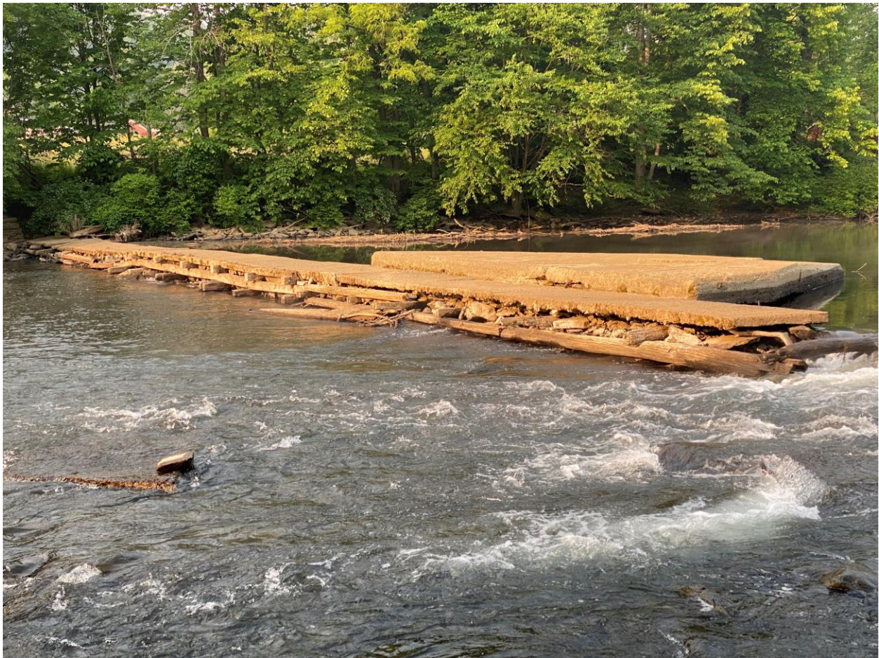
Figure 42: The Existing Dam has not been repaired since its most recent failure, which occurred sometime between 2013-2015. The dam appears to be constructed of timber and rock with a concrete layer. Given the current condition and construction of the dam, it is unlikely that repairing the dam will serve as a sustainable solution that would meet the community's needs.
