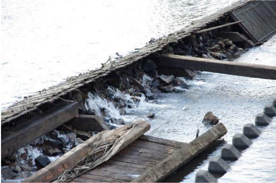
Figure 45: In the September 2016 failure of the Raftsman Dam, a 60-foot section of the dam broke off. The dam appears to be timber framing filled with rocks and additional timber, with a concrete pad below. Photo from Courier-Express Article.
