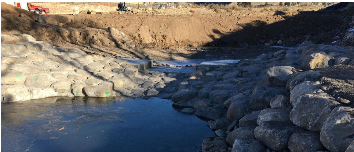
Figure 38: This structure, dewatered and under construction, shows what S 2 O designed whitewater structures look like under the water surface - the center low flow notch channelizes the river to get the most out of available flow, and interstitial spaces between boulders aid in fish passage through the structure at all water levels. The next “stair step” up is to accommodate medium flows, and higher flows rise along the grouted boulder slopes of the structure towards the banks.
