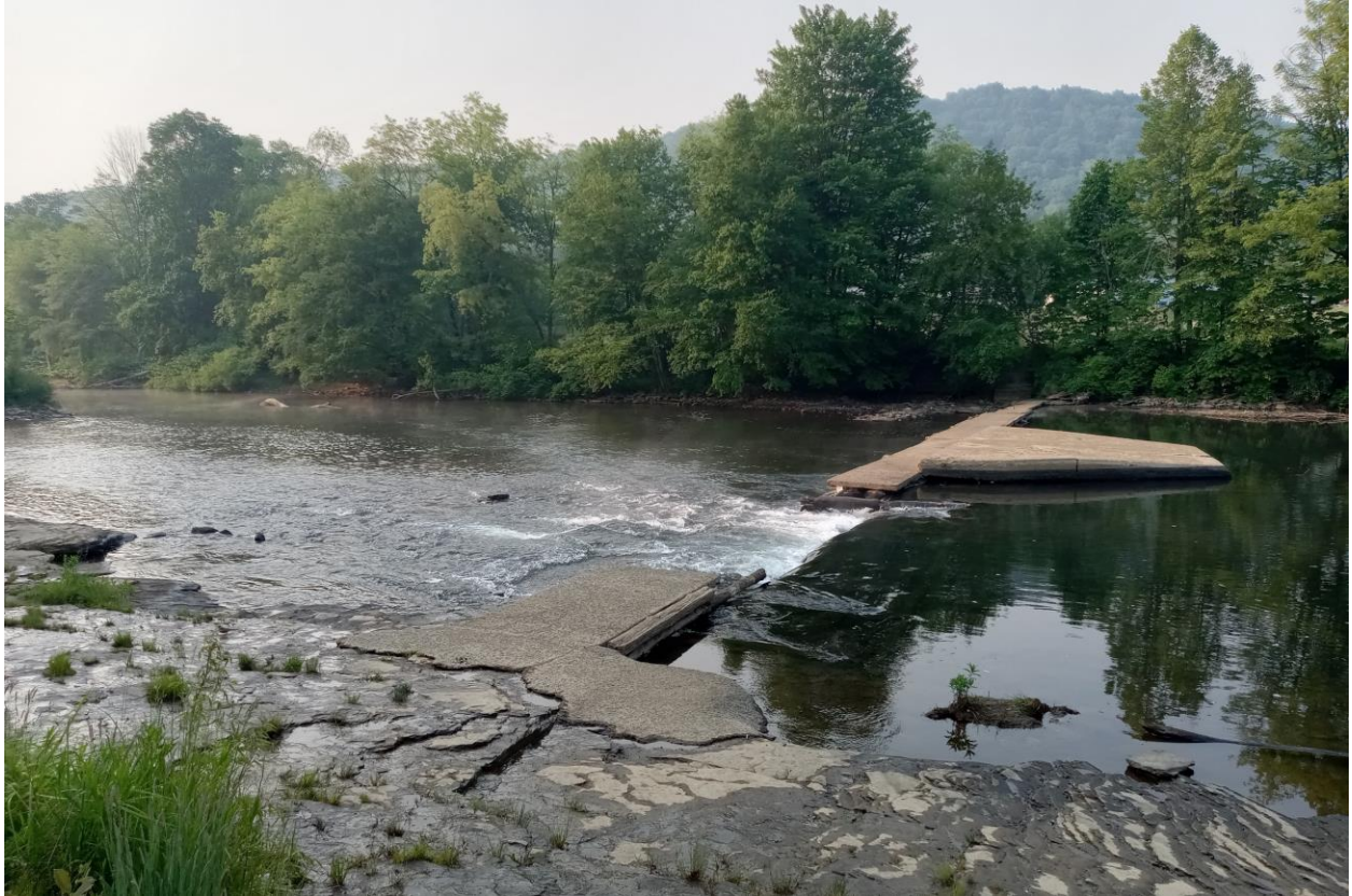
Figure 18: The failing low head dam is the subject of a conceptual design for removal and replacement with a whitewater structure.
