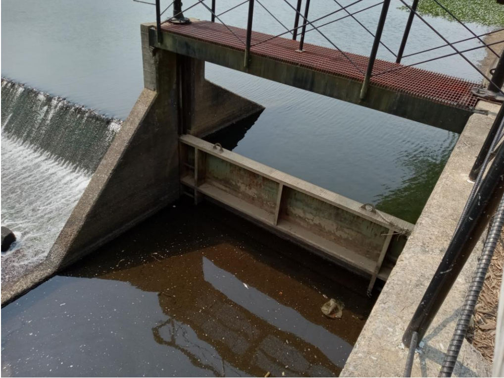
Figure 32: The river left side of the dam features a manually operated sluice gate within a concrete structure.
